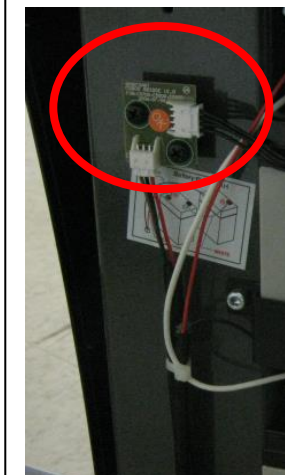
HTR sensor wires
